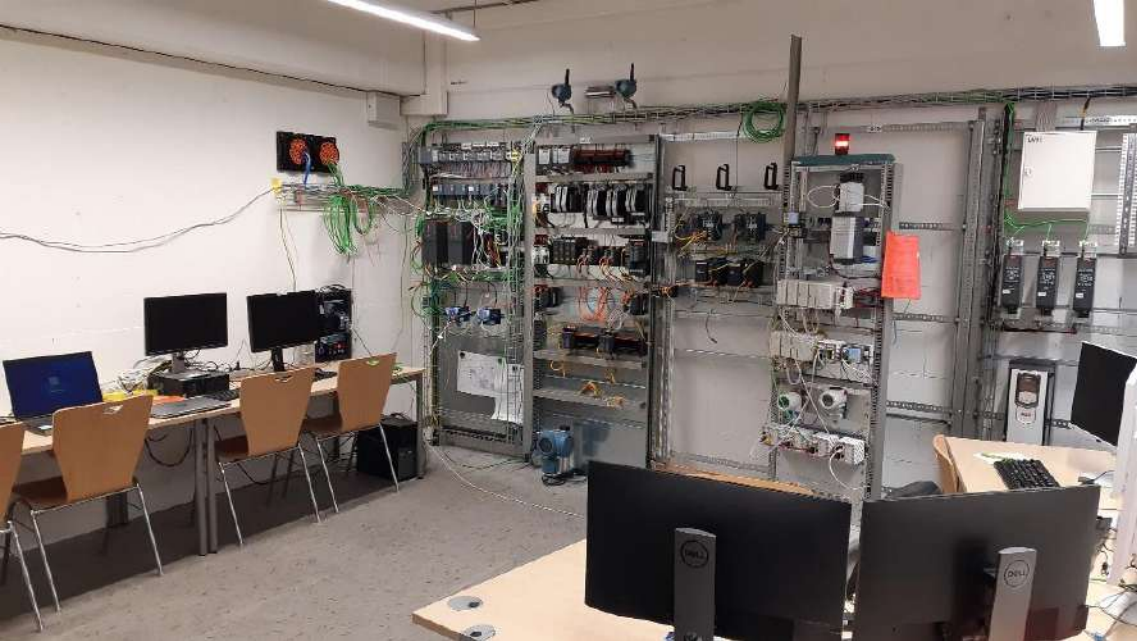
Control Level with ABB, Emerson, Honeywell and Siemens DCS
