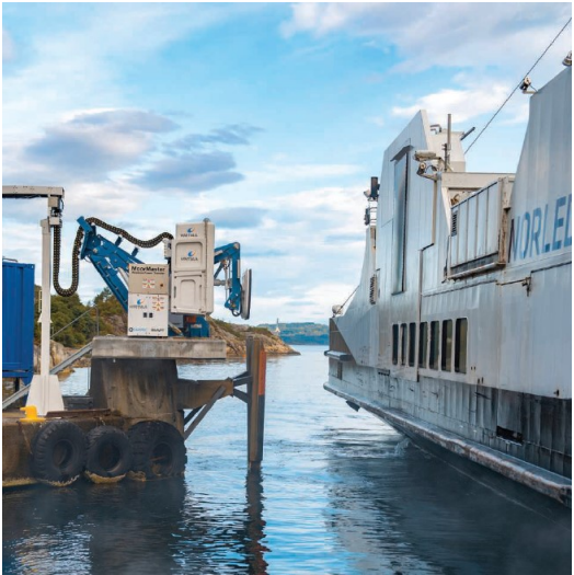
The Wärtsilä inductive charging system for charging the MF Folgefonn (Source: Wärtsilä)
