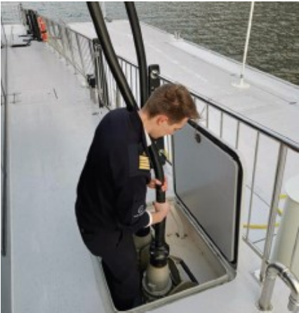
Manual connection of two cables for charging (Source: Severin Synnevag)
