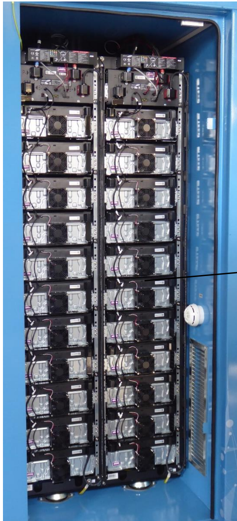
Battery Equipment Room
