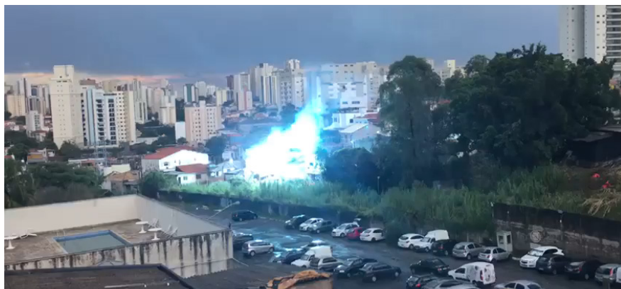
Figure 2. Sustained power arc (South America) because a cable short circuit current could not be interrupted.
