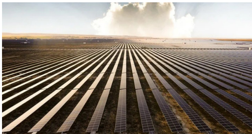
Figure 4. 1.35GW solar PV plant Konya Karapinar (Turkey).
