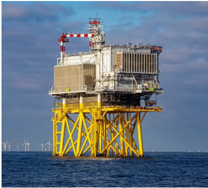
Figure 5. 700MW TenneT offshore transformer substation.
